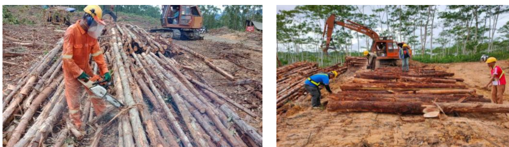
In the landing area, the full length is cut into 4-meter length.
